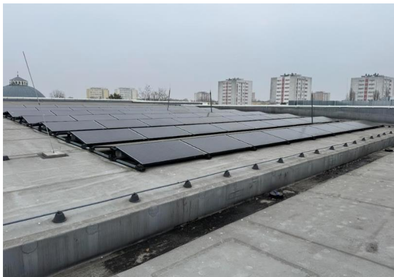
Photo 2. Photovoltaic panels installed on the roof of the Aqua Toruń complex. Toruń, 12/03/2025. Source: Author.
