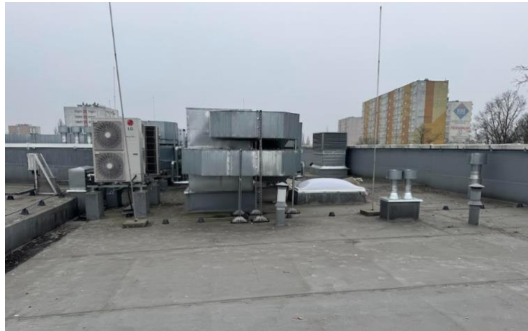
Photo 4. Rooftop heating and ventilation installation at Aqua Toruń after modernisation. Toruń, 12/03/2025.
