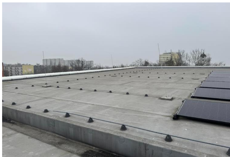
Photo 3. Roof space at Aqua Toruń where further PV modules could not be installed due to lack of funds, Toruń 12/03/2025; Source: Authors
